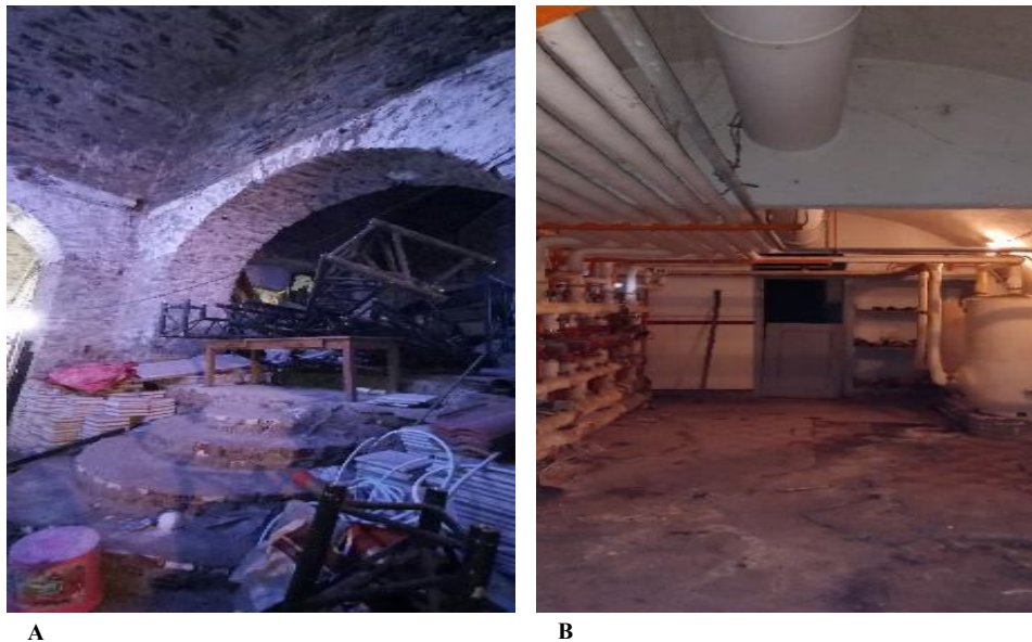
Figure 20: Some obstructed and unsafe areas not adequately covered by lasergrametry. (Source: Author, 2022). A- Cluttered and abandoned space; B- Underground boiler areas.
