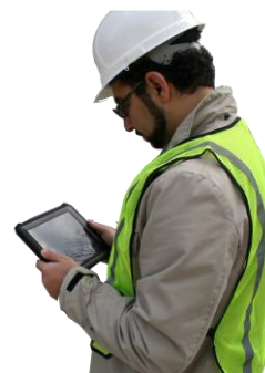
(c) Safety manager interacts with workers using the drone and through the iPad
